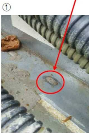
<Leakage found on Sept. 11> ① Pencil-size leakage occurred from the bolt hole. * No damage or dent was found.
