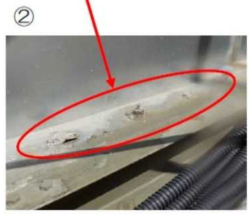
<Leakage found on Sept. 12> ② Leakage at a rate of one drop per 10 seconds from the bolt section * No damage or dent was found.
