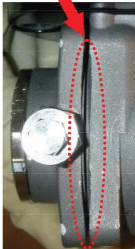
Condition of the bonnet flange (top) Note: The flange is slightly swollen and the O-ring is projecting out of the flange.
