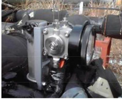
External appearance of the affected differential manometer Note: No traces of damage (scratches, deterioration, etc.) on its exterior
