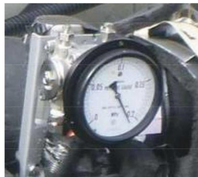
Reading of the affected differential manometer when leakage occurred Note: The indicator is off the scale.
