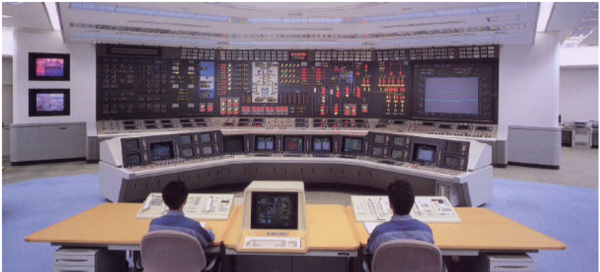
Fig. 12.1 Main Control Panel of Kashiwazaki-Kariwa Unit-6 (ABWR) of Tokyo Electric Power Company
